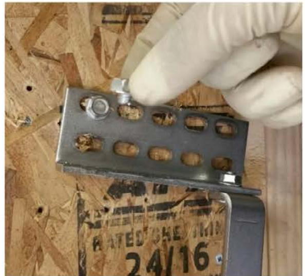
Figure 3b. Typical Failure Mode
