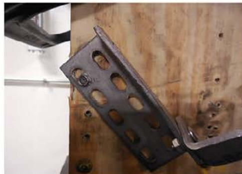
Photo 12: Failure of Screw Head
