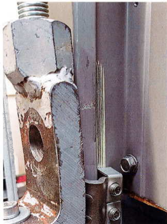
Figure 2b. Typical failure mode.
