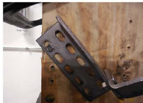
Photo 12: Failure of Screw Head
